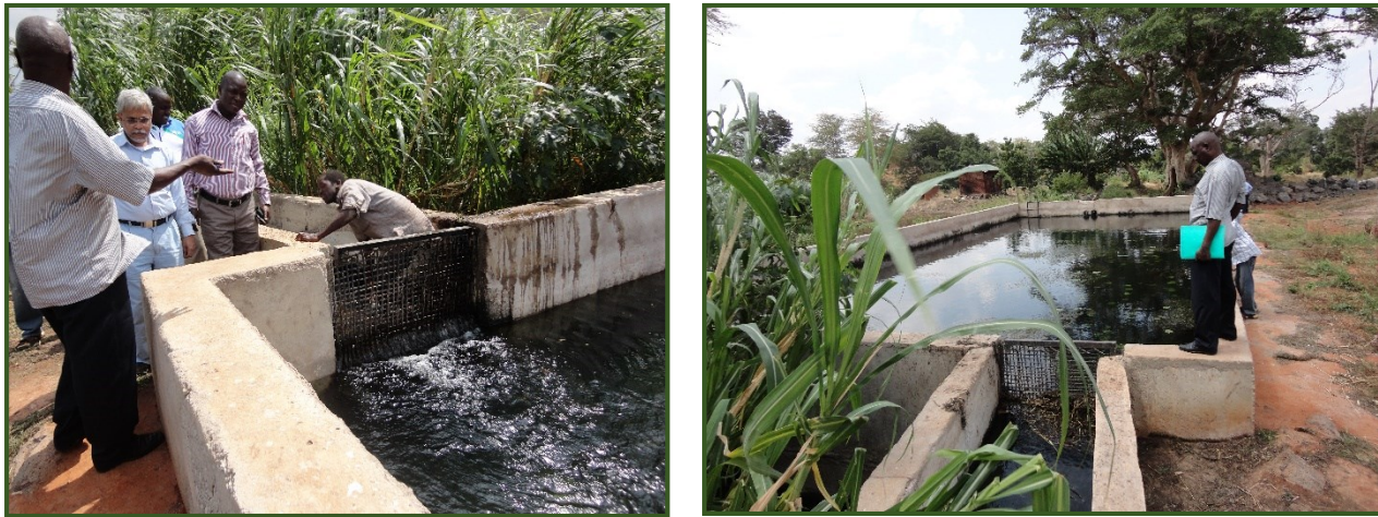
Figure 1: Inlet for the Drip Irrigation System
